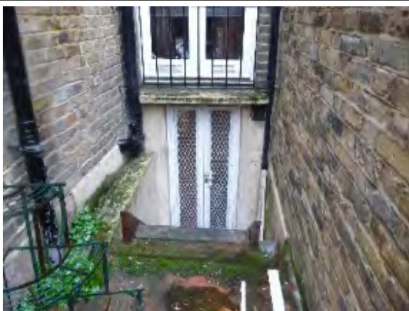
5. Subterranean rear doors - area very wet
