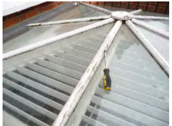
4. Rotten frame to lantern
